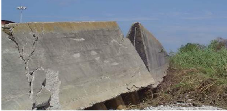
Figure 4.2. Local Failure of one panel (IPET V-14-64)
