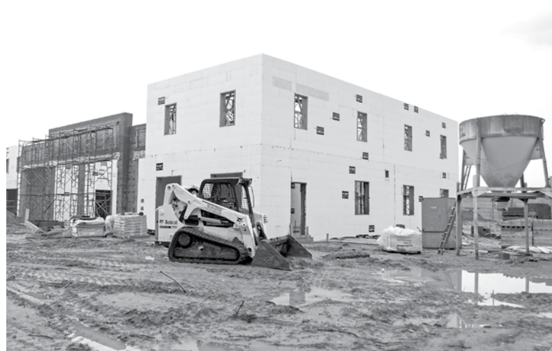
Construction for Fire Station No. 1 on McElroy Drive is seen Monday. LOGAN KIRKLAND | The Daily Mississippian
