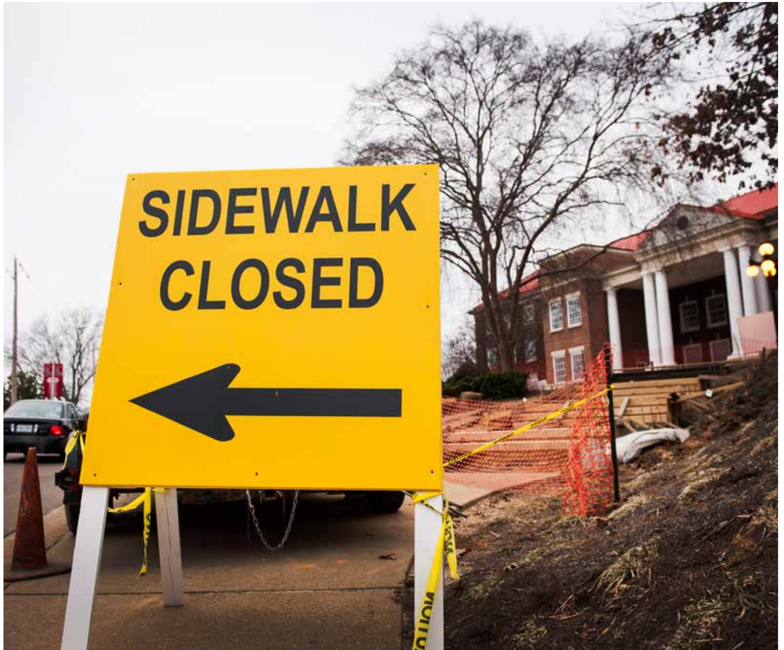
A closed sidewalk is seen by Martindale on Monday. The construction entails adding new steps and a railing.
