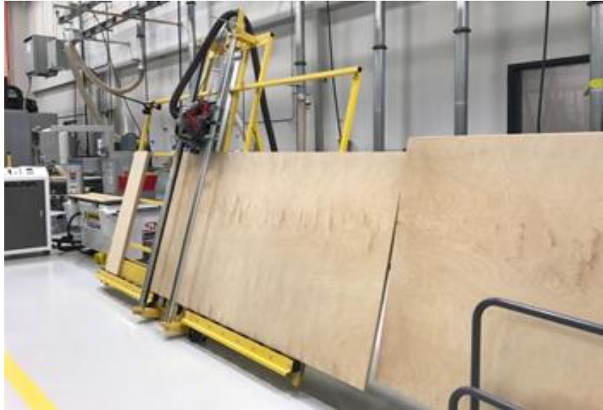
Figure 35 - Wood Supply to Panel Saw
