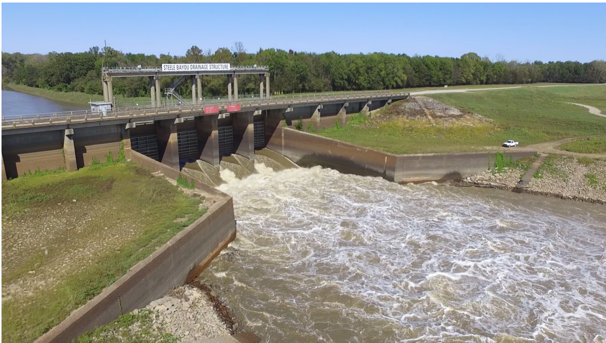
The Steele Bayou Control Structure situated at the bottom of the Yazoo Backwater Area
