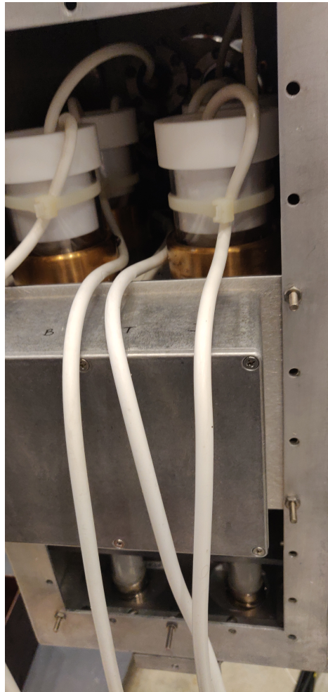
Figure A.8: Potted RF resistors after being installed in all of the eight quadrupole systems, the white cables connect the resistors to the transformers that are used to provide more power and hence more CBO reduction
